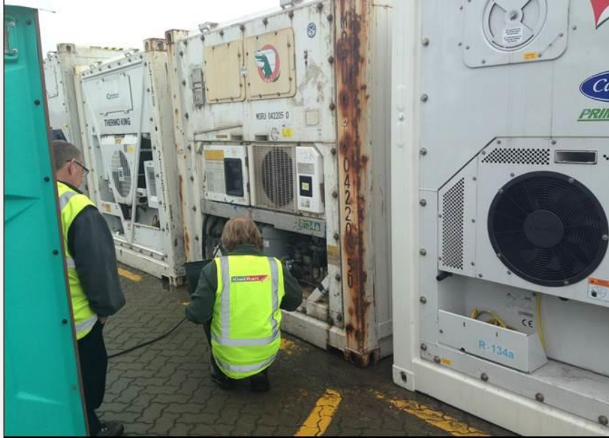
Figure 7.6 – Shipping container in rail marshaling yard in Christchurch
